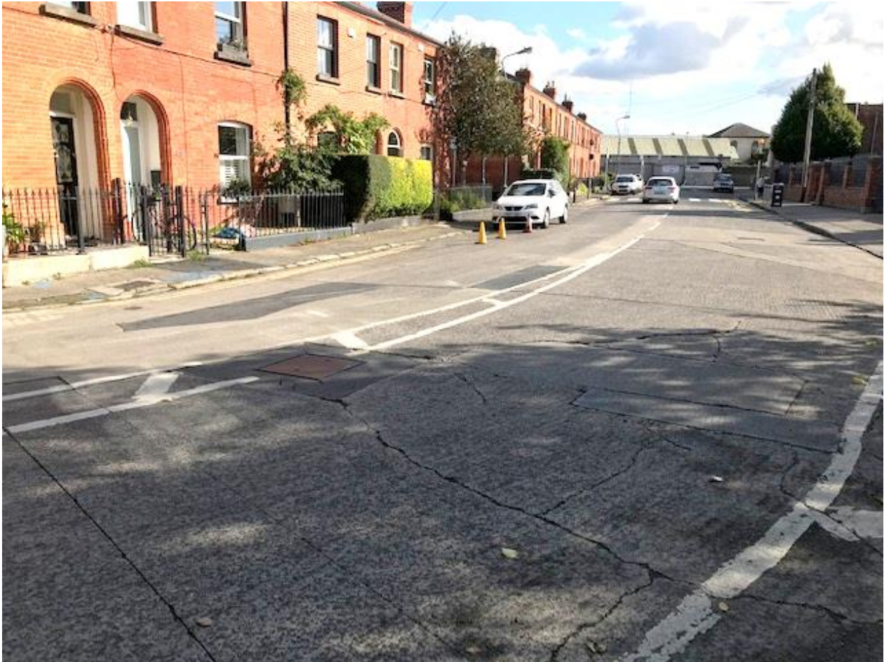
Figure 2.3: Condition of road surface
